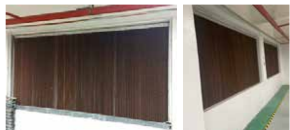
Water cooling system in operation floors
